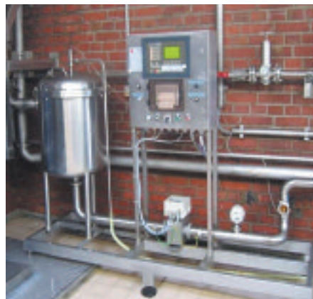
Officially calibrated reception system with flow meter, operator terminal and voucher printer
