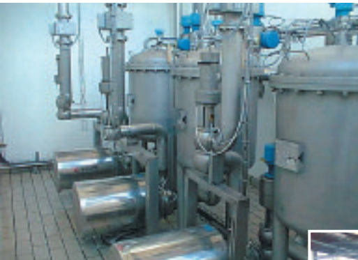
Self-filling reception equipment in the cellar
