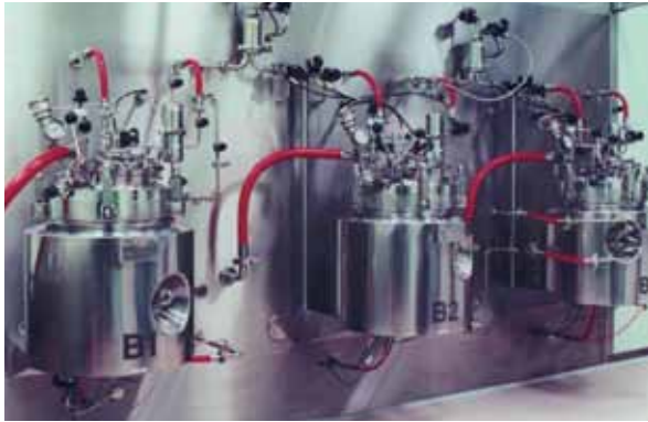
Clean room partition wall with integrated preparation vessel
