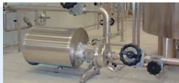
Loop circulation pump
