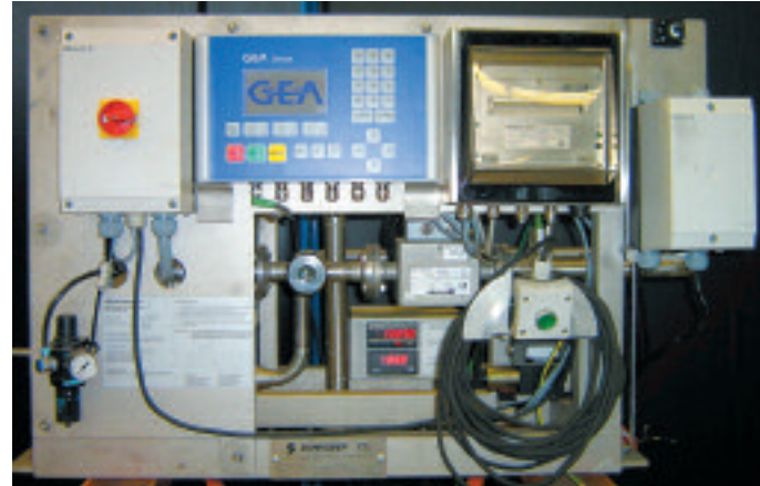
Tanker measuring unit with the new ZEVODAT-flash data capture system
