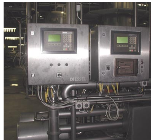
Figure 3: DI-LIQUIZ™ twin system in a blending plant. Photos: GEA Diessel
