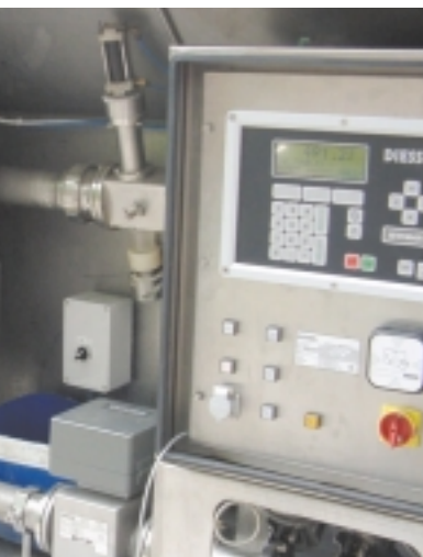
Officially approved metering apparatus with control unit and Zevodat-M data acquisition unit
