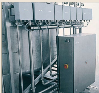
Metering technology for the filler lines
