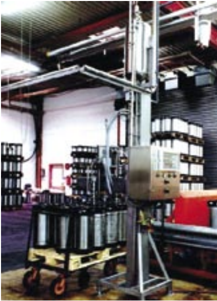
Figure 6: Post-mix filling plant
