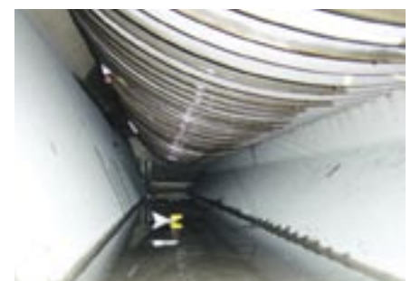
The flow channel in the bottom pre-soak segment. The high turbulence of the flow gives the dirt involved no opportunity to collect. Photo: Kronen AG
