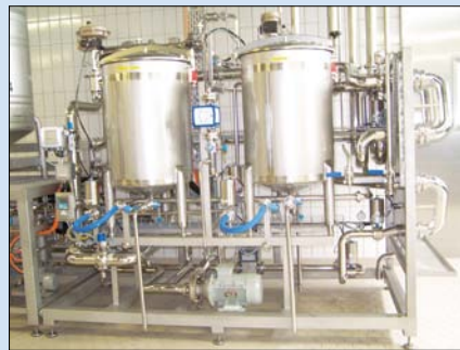
Figure 2: Permanently installed component tanks for the pre-dissolution of dry ingredients
