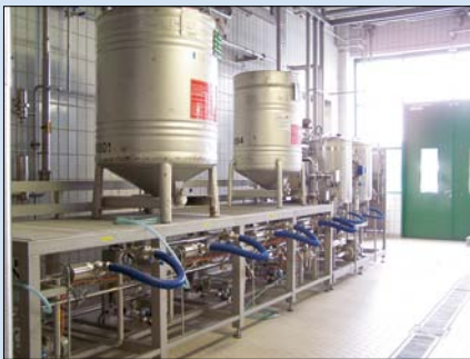
Figure 1: Beer blending unit with four container positions and two permanently installed dissolving and storage vessels
