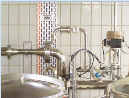
Figure 4: CO 2 dosage; injector and regulating valve
