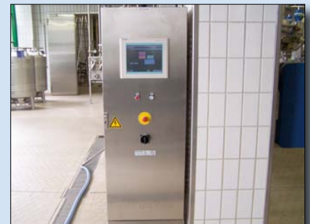
Figure 6: Control cabinet with graphical operating panel
