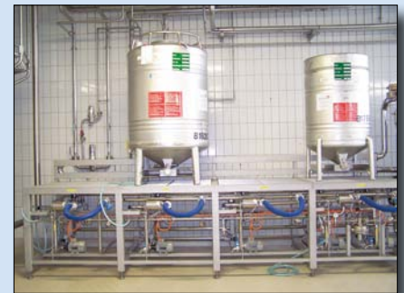
Figure 3: Positions for the swap tanks with the gravity lines supplying the concentrates to the individual dosage lines
